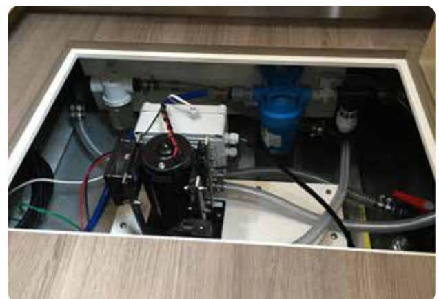
Watermakers installed in various positions on the boat
