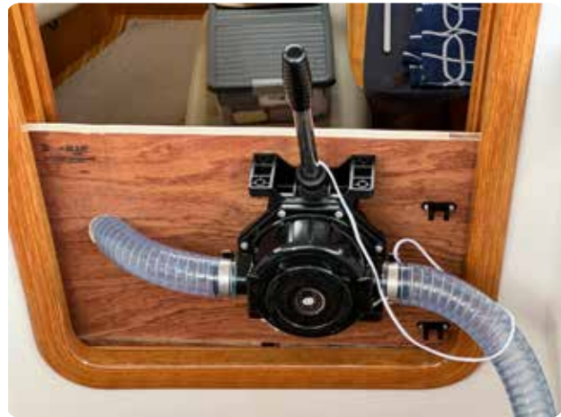
Pump fitted to a spare washboard on a Hallberg-Rassy
